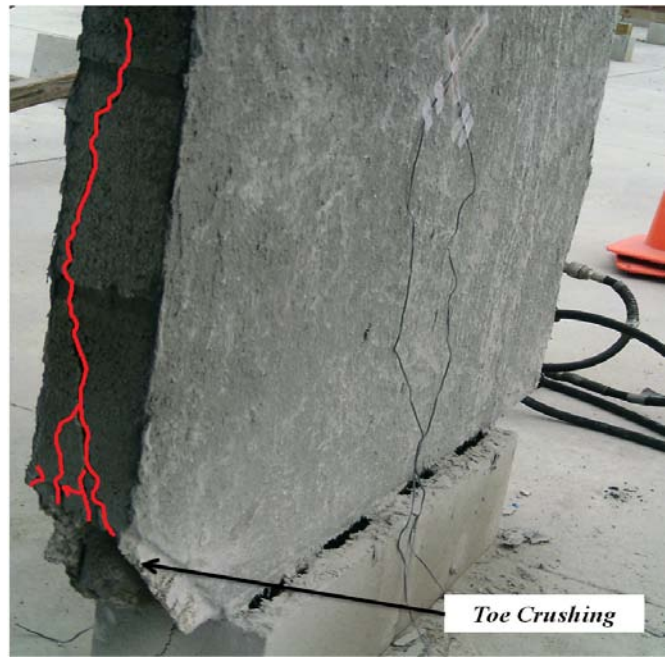
(Crack line enhanced)
